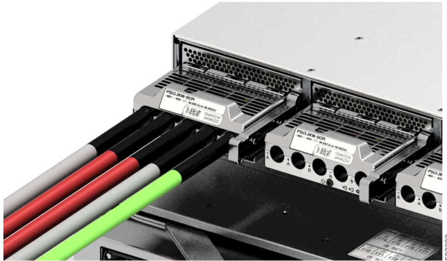
Figure 46: Close Terminal Block Cover
