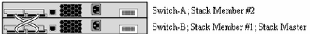
First Switch Stack Consists of Switch-A and Switch-B
