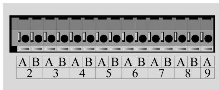
Close-up of Front Panel Terminal Strips
